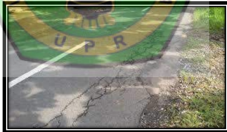
Gambar 2.3 Retak Acak ( Irregular Crack )
