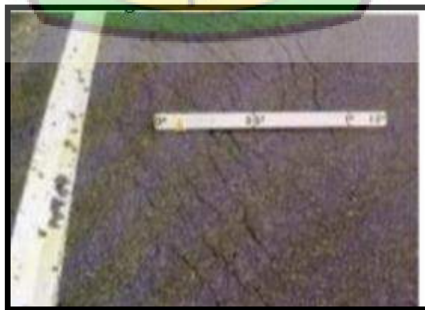
Gambar 2.39 Patah Slip ( Slippage Cracking )
